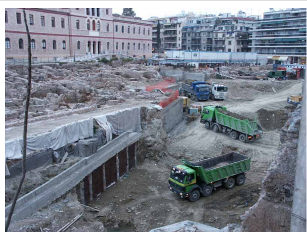
Earthworks in the archaeological site in Makrygianni, during the construction of the museum.
